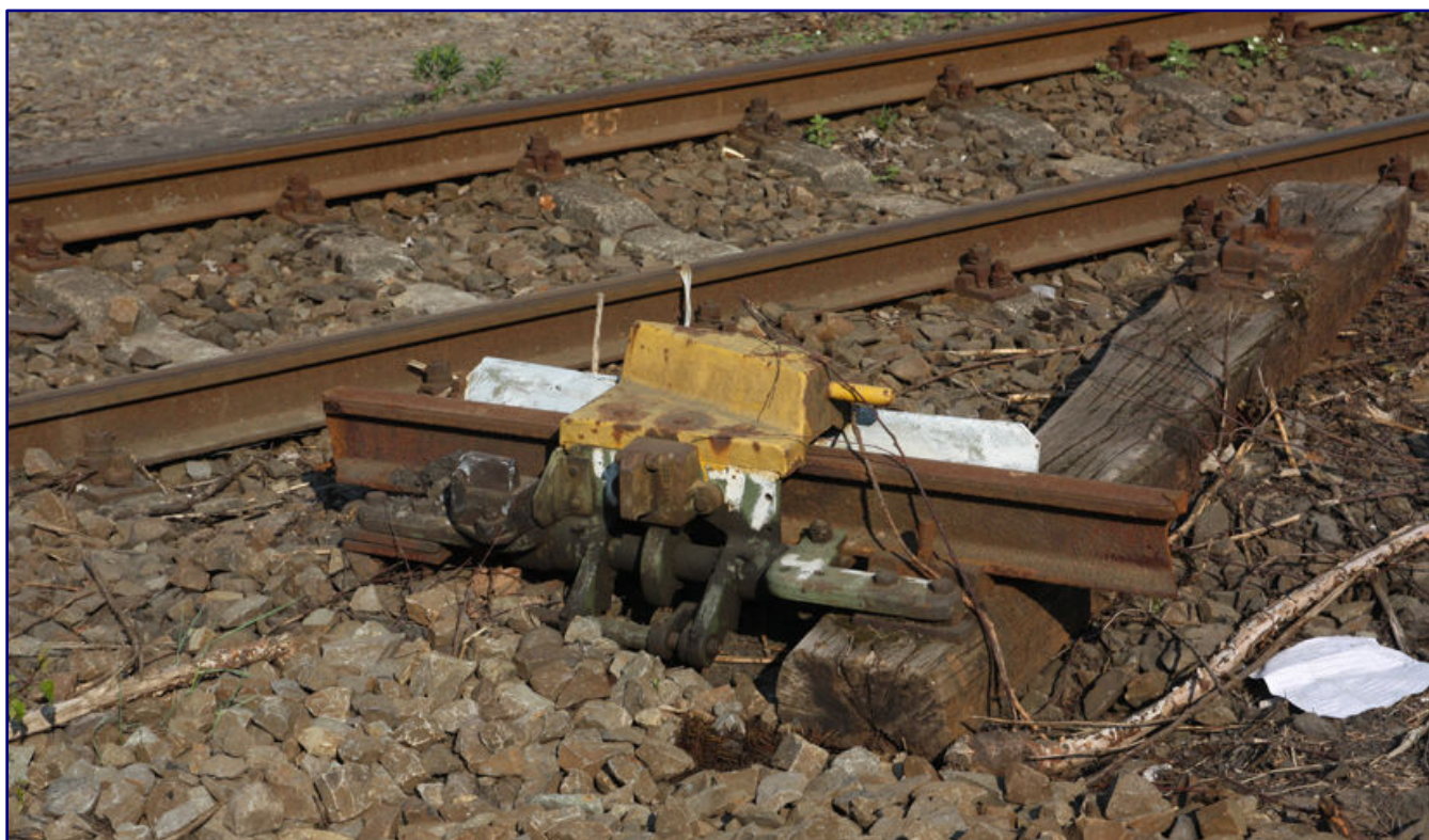
For almost two years, many parts of the signalling technology lay around rusting in the Opladen station area, which had not yet been converted (photo above). Leverkusen-Schlebusch station used to have a number of sidings. After the dismantling, the remnant of a track closure lay here in the gravel bed for years (photo below).
