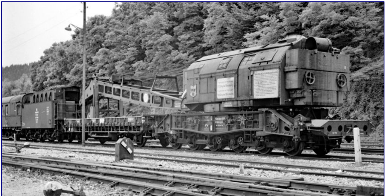
On 13 July 1968, the 57 to. crane “München 6664” stands in Gaildorf-West station to replace bridge parts on the Kocher Bridge. The photo also shows the supplying tender 2'2' T 34 and the staging car for the crane personnel – a former “Hechtwagen”. Photo: Wolf Schneider, Collection Eisenbahnstiftung
